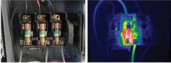
FAULTY / CORRODED FUSES
